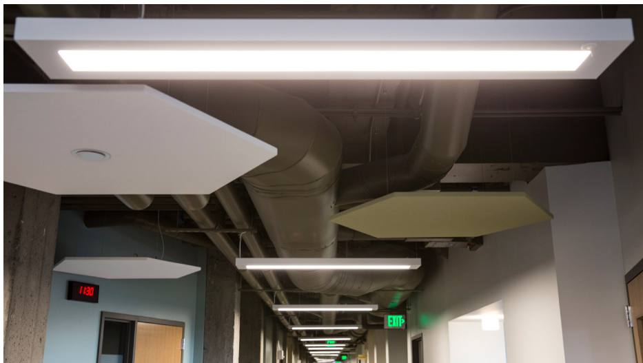
Enlighted Luminaire Level Lighting Controls installed in the Pacific Tower building in Seattle, WA.
